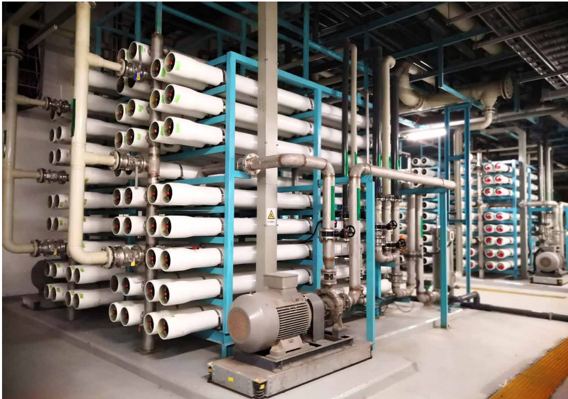
Reverse osmosis water filtration system
