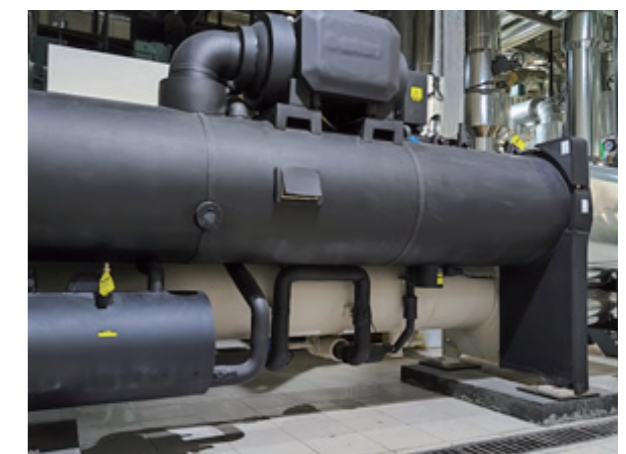
Newly-assembled 150-RT chiller
