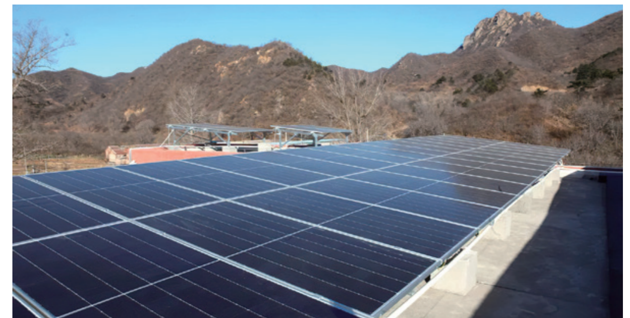
BOE launches the photovoltaic power generation project to support villages with weak collective economy in Dazhuangke Township, Yanqing District, Beijing
