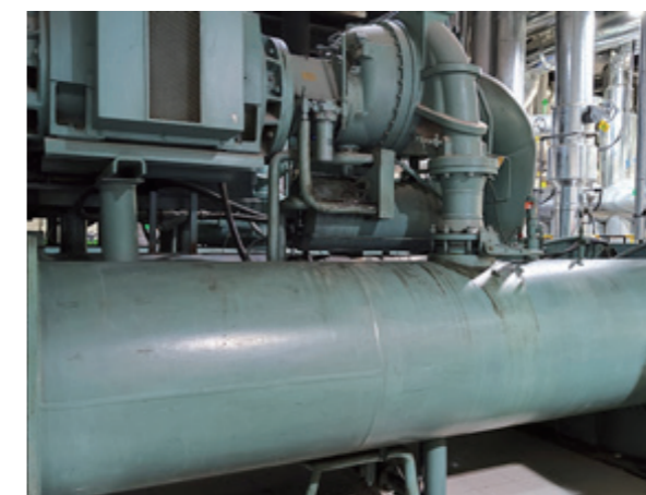
Existing 750-RT water-cooled chiller
