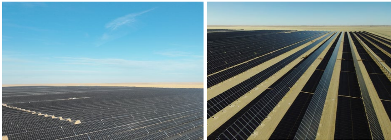
200 MW integrated demonstration project for animal husbandry, photovoltaic, and energy storage in Sunite Right Banner, Xilin Gol League, Inner Mongolia
