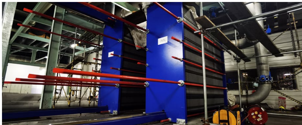
Tap water preheating transformation project for BOE Hefei Gen 10.5 TFT-LCD production line
