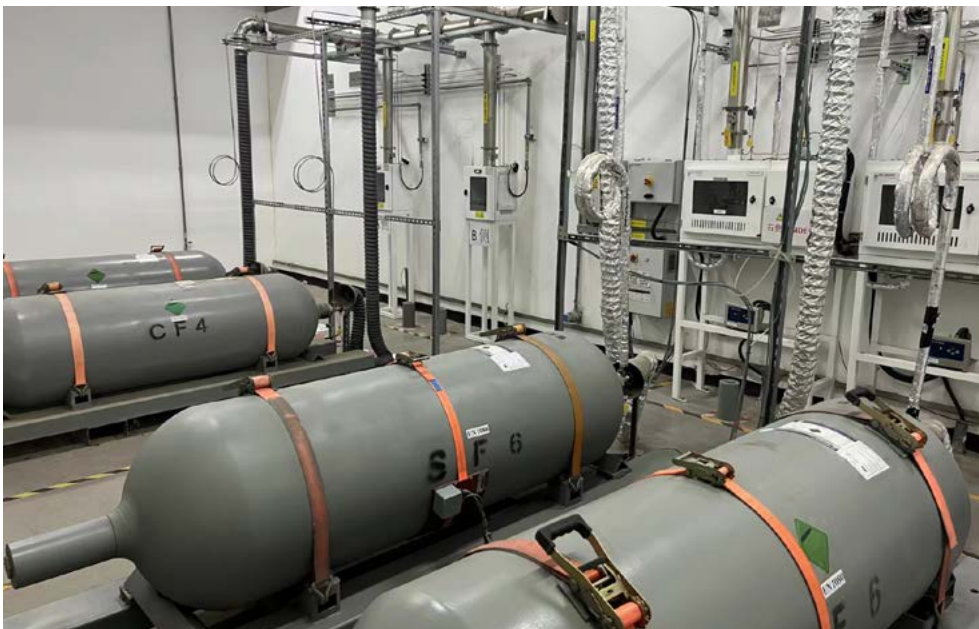
Normal Gas Supply in the Sulfur Hexafluoride Gas Supply Room at the BOE Beijing Gen 5 TFT-LCD Production Line, with Cylinders Securely Fastened and the Site Equipped with Emergency Ventilation Devices and Other Safety Measures
