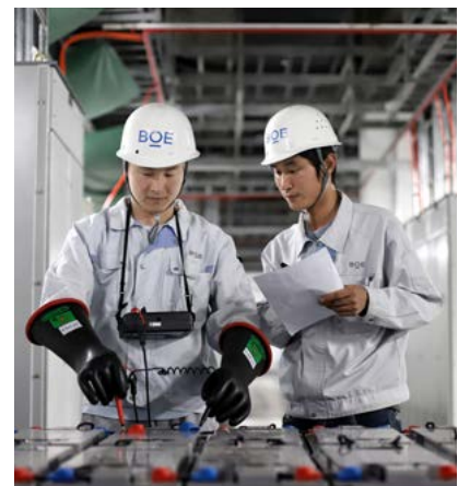
Employees of Electricity Department Clad in PPE during the Inspection of the Power Distribution Room
