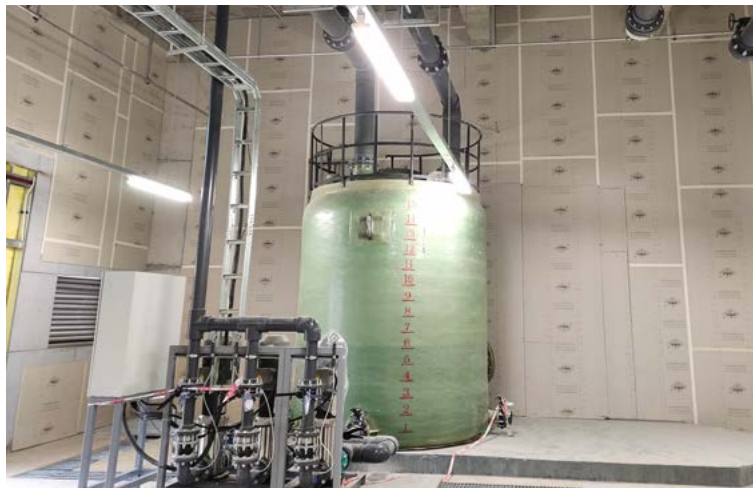
Wastewater Cleaning and Recycling Installation at Chengdu BOE Vehicle Display Technology Co., Ltd.
