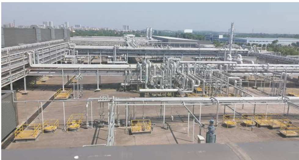
Wastewater Treatment Installation at BOE Wuhan Gen 10.5 TFT-LCD Production Line
