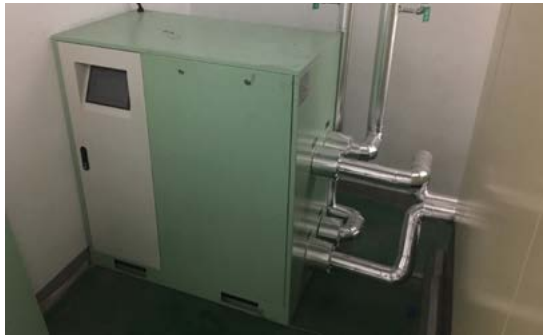
Waste Heat Recovery Heat Exchanger Installation at Hefei BOE Vision-Electronic Technology Co., Ltd.
