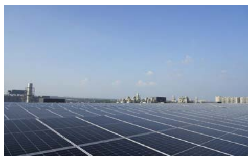
Rooftop PV and PV Carport Project at BOE Wuhan Gen 10.5 TFT-LCD Production Line
