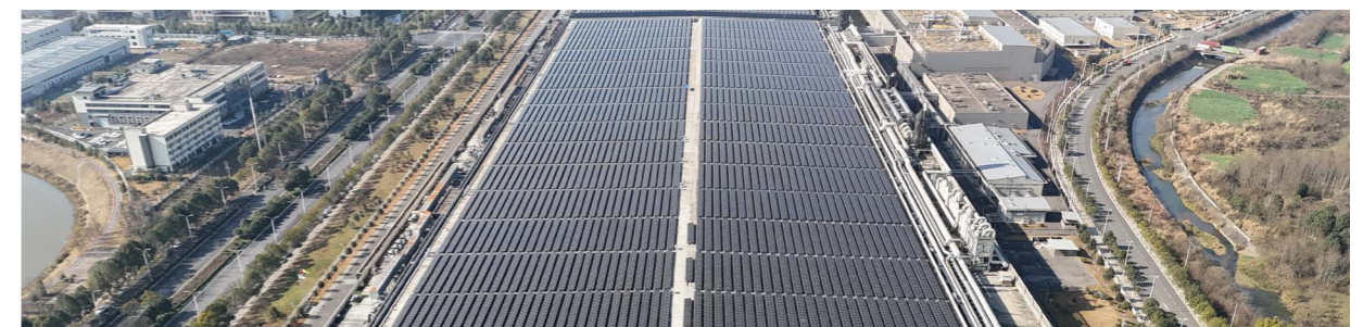
● Rooftop Photovoltaic Systems
