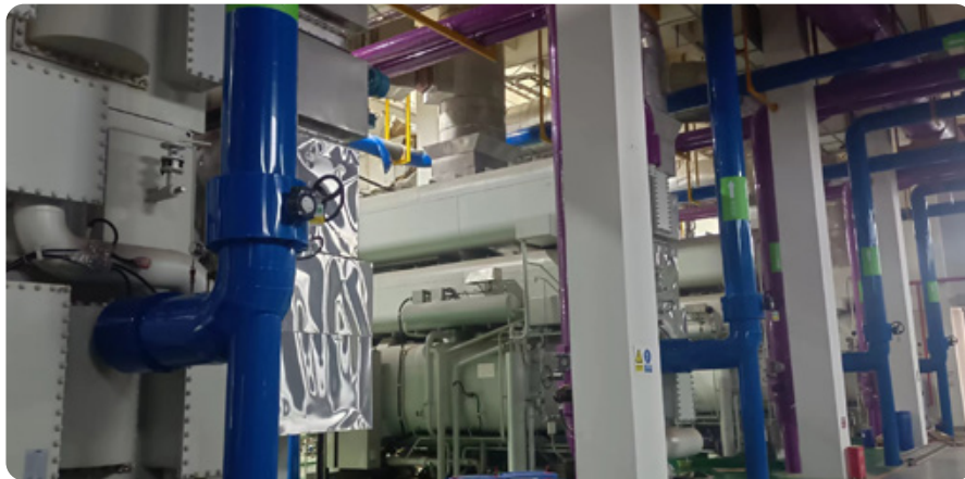
Natural Gas Distributed Energy Station Units
